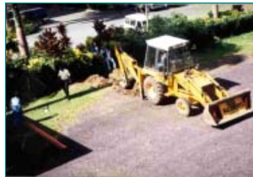
Figure 5: ITC - Civic Towers Fibre optic connection
